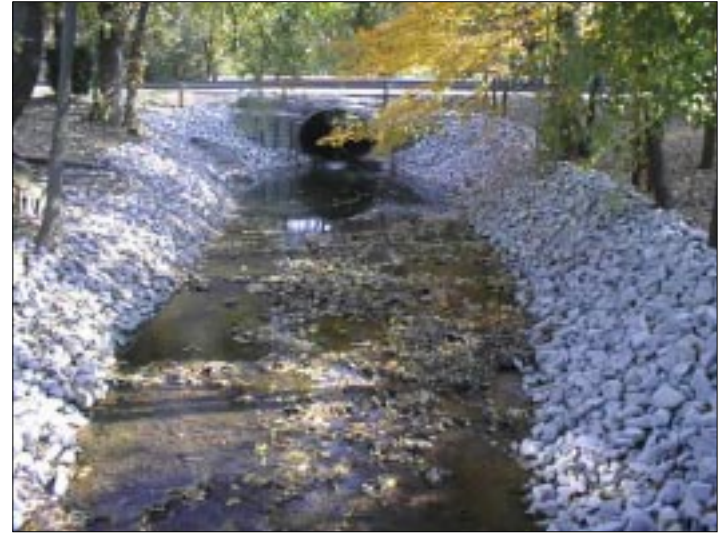
After stabilization, the stream bank is armored against further undercutting with rip rap.
